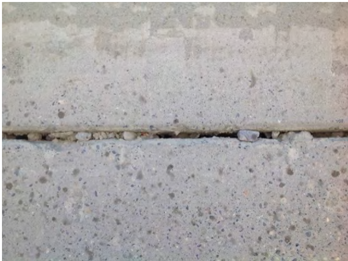
sealant missing and gravel getting between the slabs
